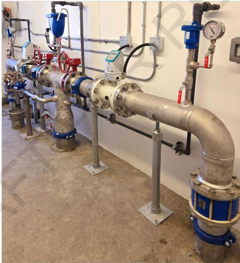
Water system infrastructure supporting the Village water supply.
